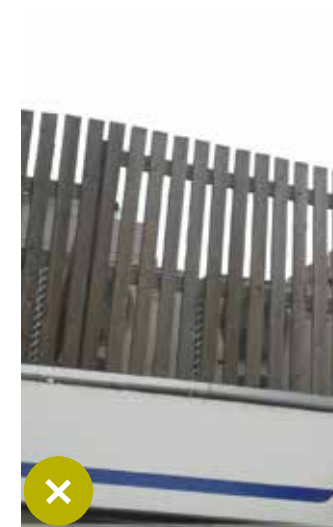
Poor plant screening
