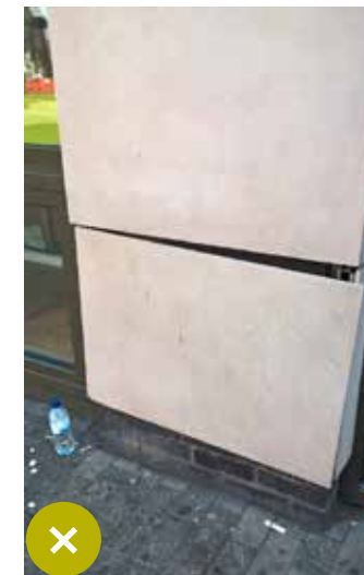
Poor construction detailing
