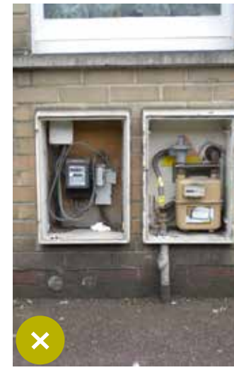
Damaged meter boxes
