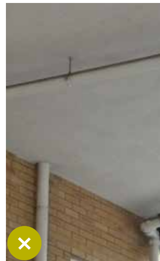
Soffit pipes unattractive
