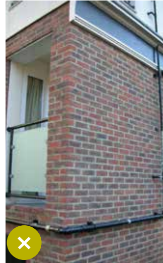
Ugly gas pipes
