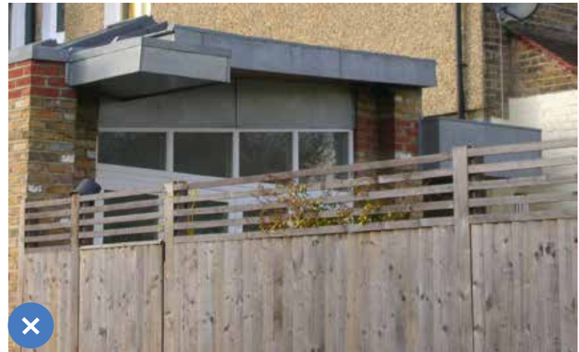
Visually obtrusive roof detail
