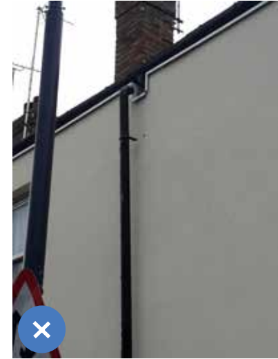
Poorly executed external insulation
