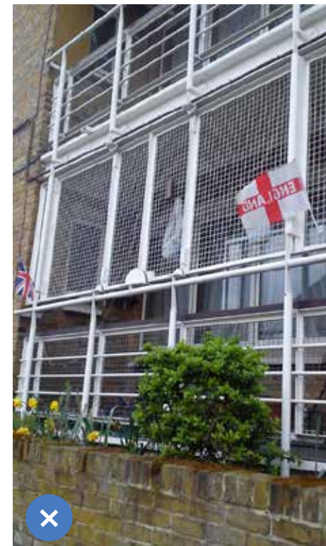
Caged balconies are unacceptable
