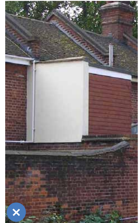
Poor closet return
