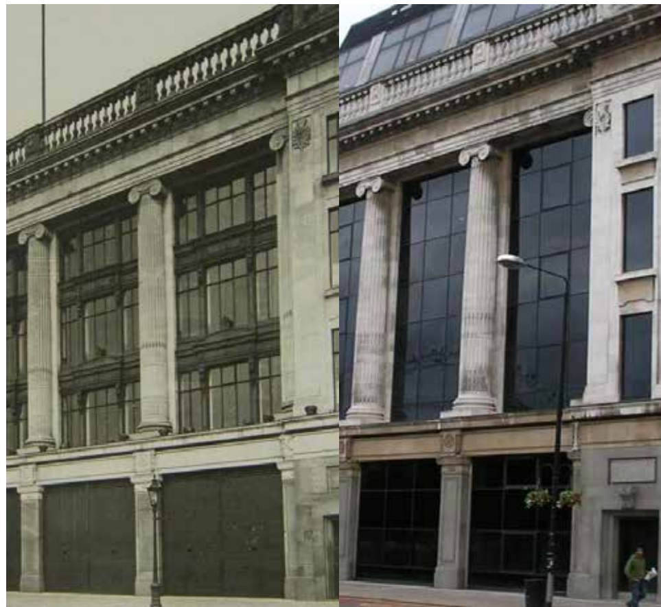
The loss of historic glazing in this façade retention has harmed the integrity of the retained façade.
